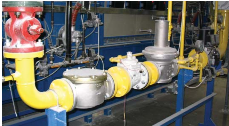
The main gas fuel train system consists of components for gas filtration and regulation with overpressure protection, as well as modular safeguard controls and fuel monitoring.
