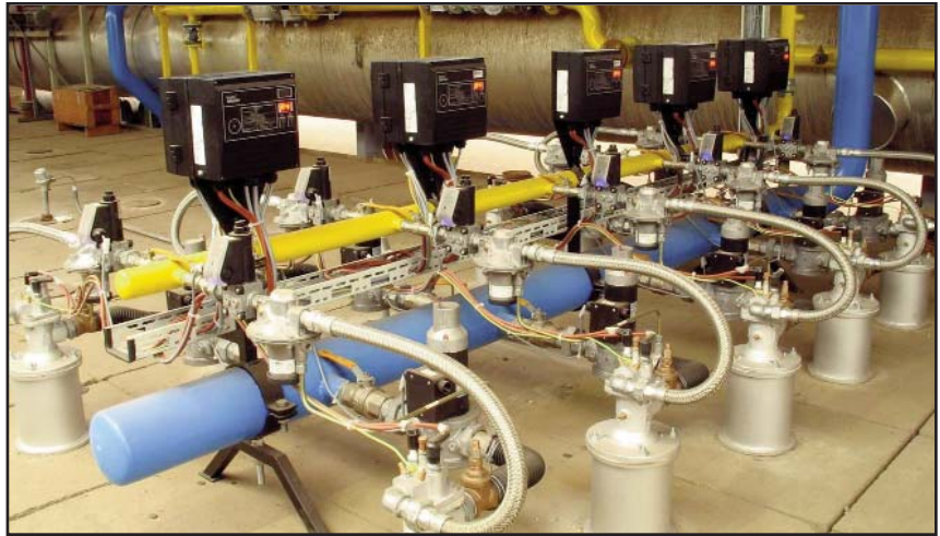
Fig. 6 - Multiburner system with locally mounted burner control units.
