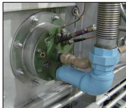
Fig 4. - Hearth level SVG burner
