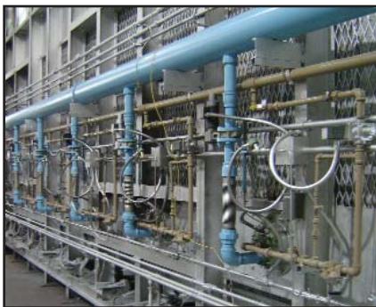
Fig. 1 - Car-bottom heat-treating furnace
